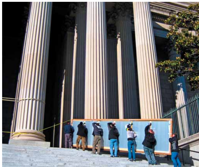
The completed frame, minus the artwork and glazing, was carried up the front steps of the National Archives, the only possible entrance to the building. The frame weighed 250 pounds at this point.
